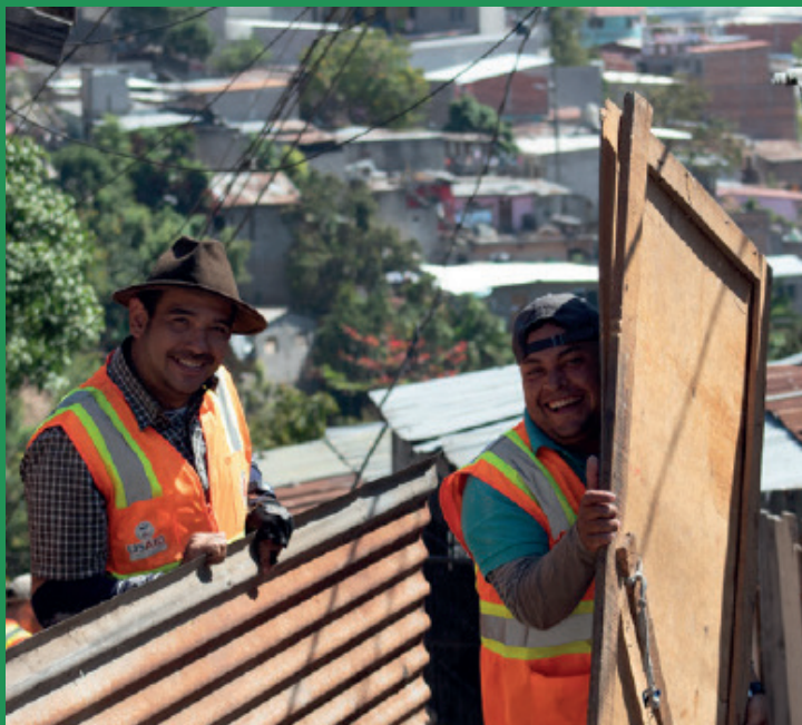
Volunteers work in the demolition of vulnerable houses vacated by families relocated from high-risk areas. (GOAL, 2018)
