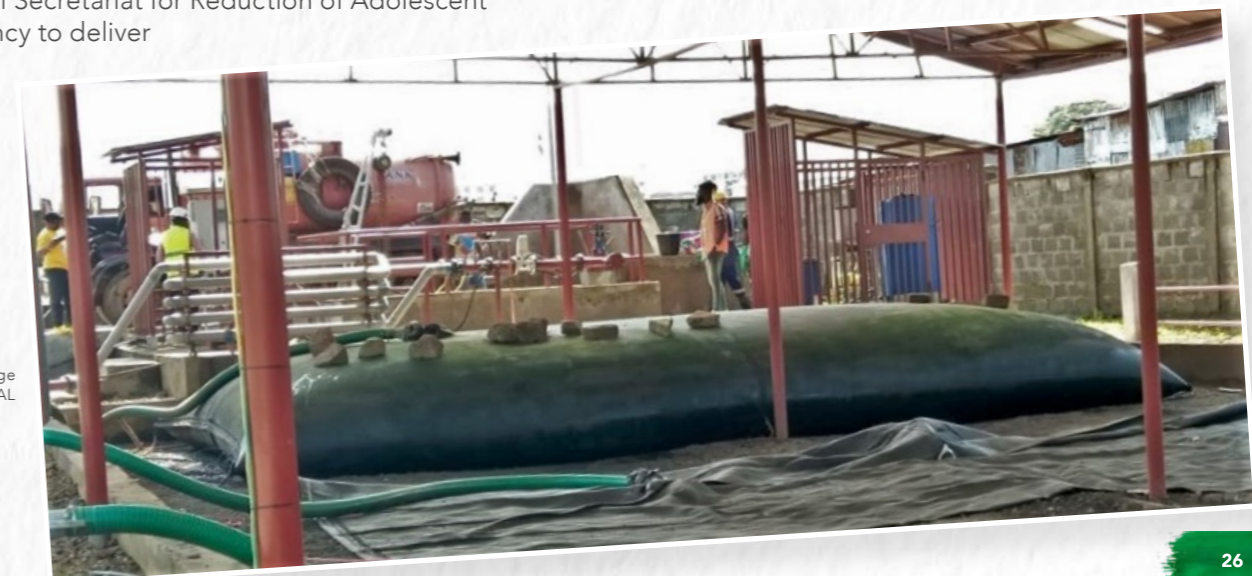
Kingtom Faecal Sludge Treatment plant, GOAL Sierra Leone
